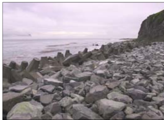
A revetment slope armored by precast concrete dolosse is topped by a rock splash apron at the airport in Unalaska (photo by Harvey Smith, Alaska Department of Transportation and Public Facilities).
